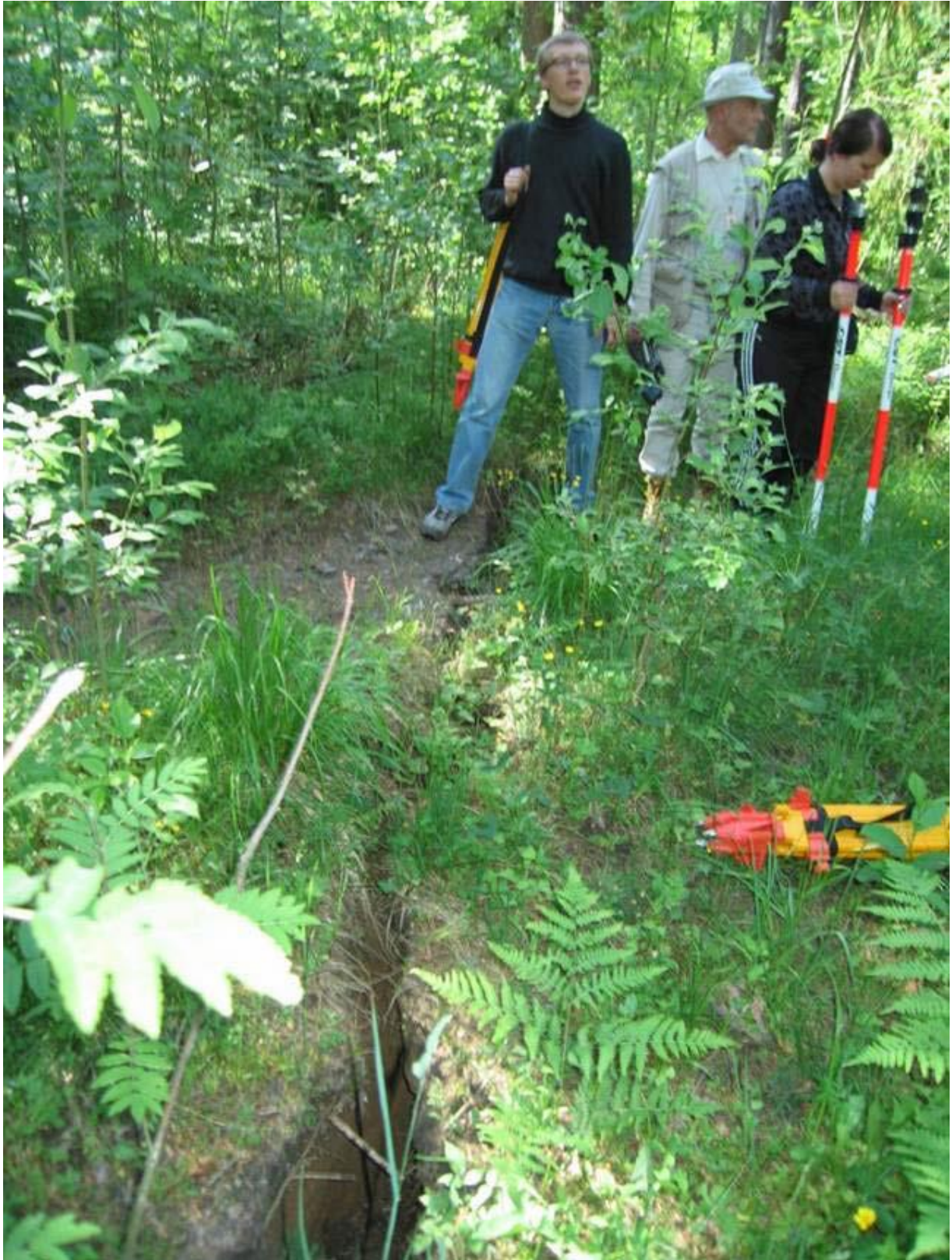
Figure 8. A considerably large surface opening above the collapse from 2008 (Soosalu, 2009).
