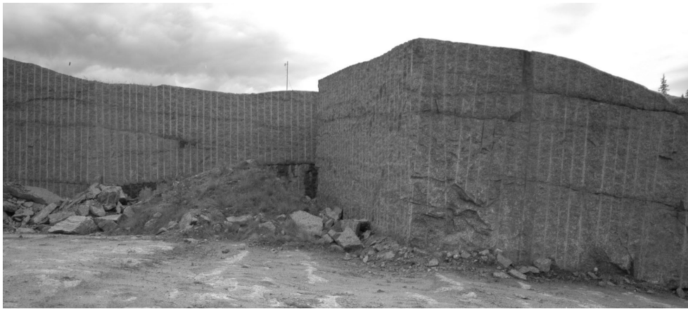
Fig. 3. Sub-horizontal and sub-vertical fracturing of porphyritic granite. Height of the bench is about 5 m.
